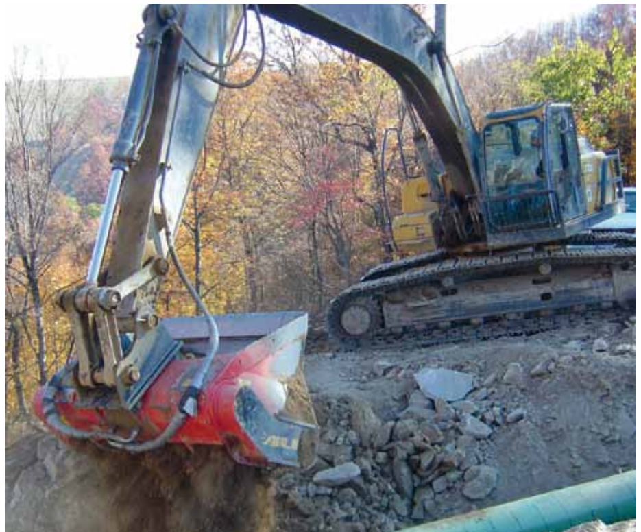
An Allu screener crusher being used on the Columbia Gulf Gas Pipeline project.
